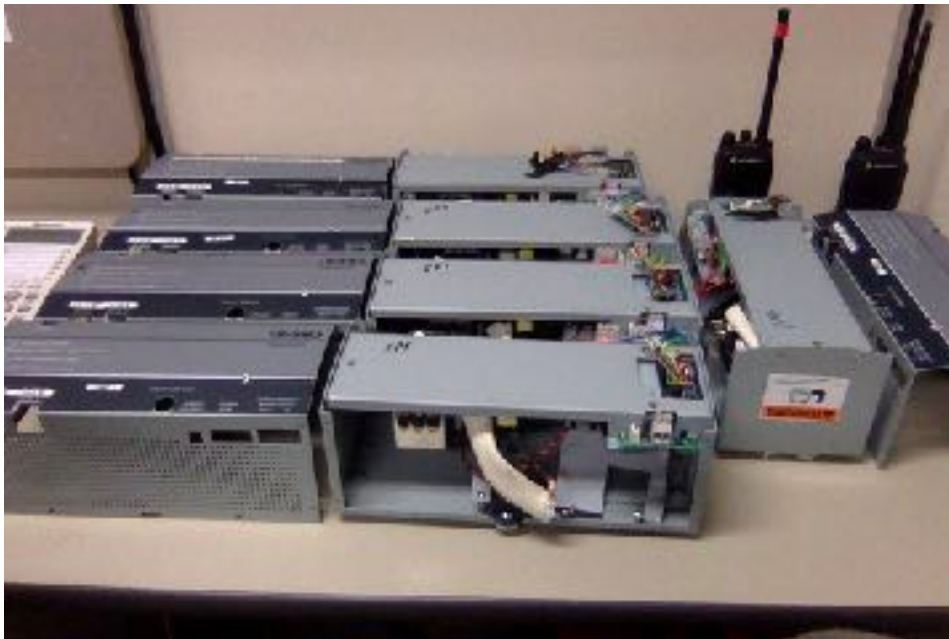
UPS Devices waiting to receive new batteries
